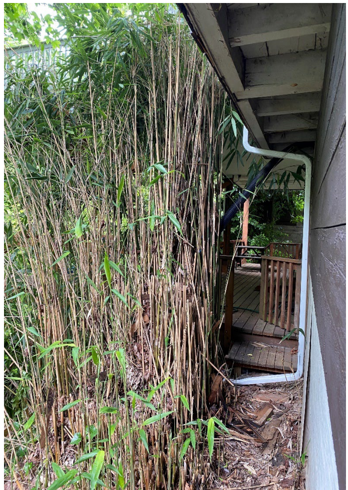
Invasive bamboo leading up to structure
