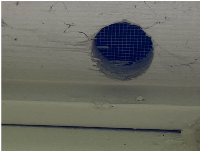
Example of 1/8 inch screening installed on attic vent openings – also known as “bird blocking”.
